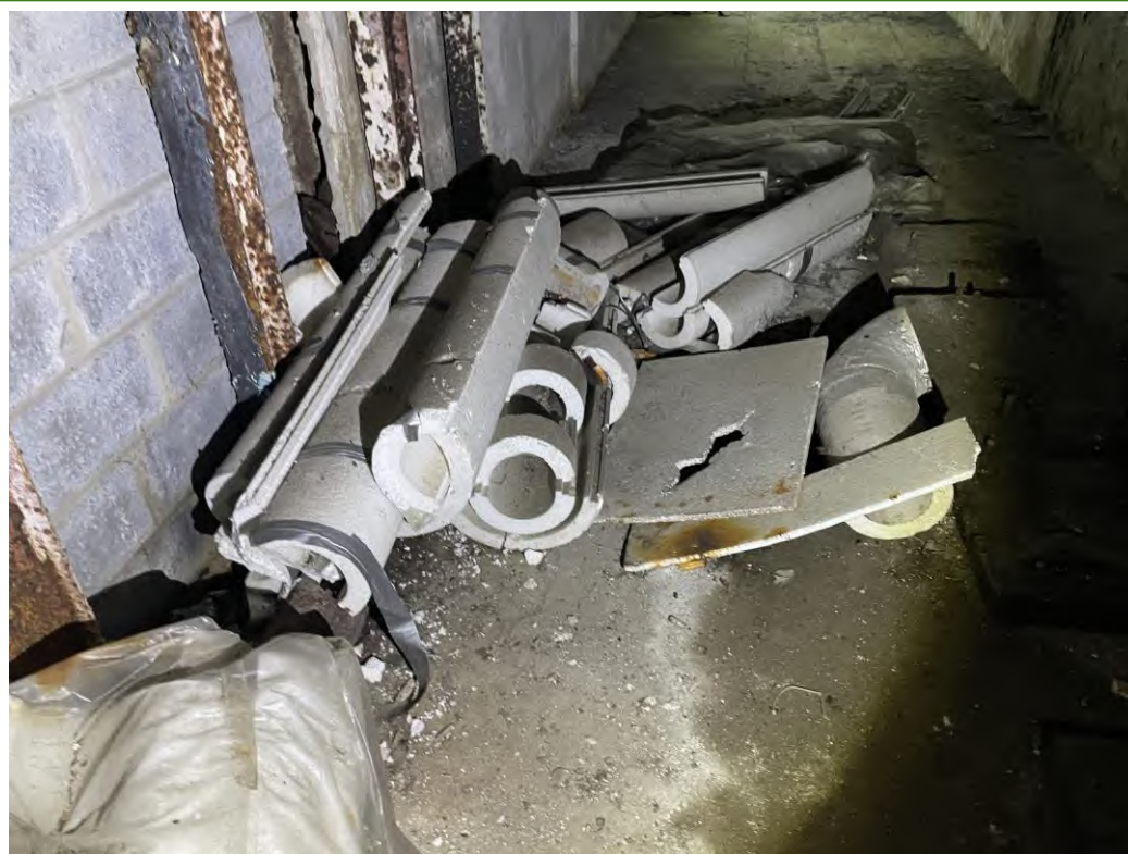
Pipework insulation in building 1
